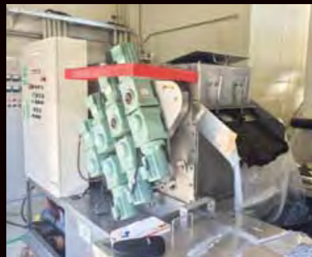
Mixed Sludge at Confectionary Plant (JD-500)
